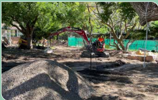
Construction of the Outdoor Classroom began in October 2025, and will be completed in early 2026.
