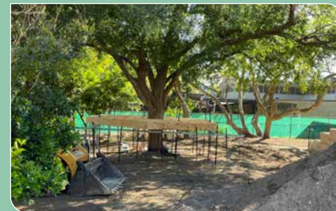
When finished, the Tree House will be connected to Possum Hill by a rope suspension bridge, offering plenty of opportunities for adventurous play.
